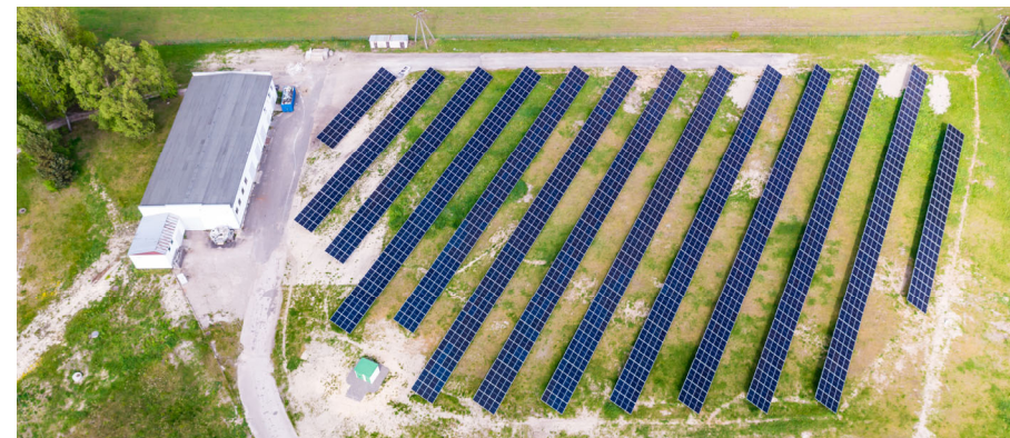
Photovoltaic system in Bilgoraj
